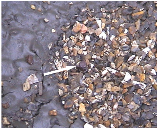
B As 10A above with nozzle excavated to show its position (arrow), just beneath the surface of the gravel layer
